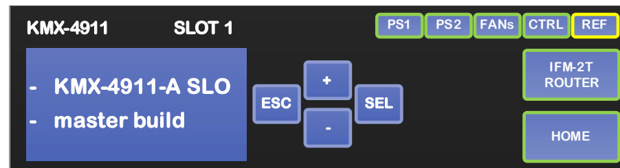
CPU-ETH3 local control panel
